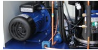
Pump P3 (3 barg) / P5 pump (5 barg, optional).
